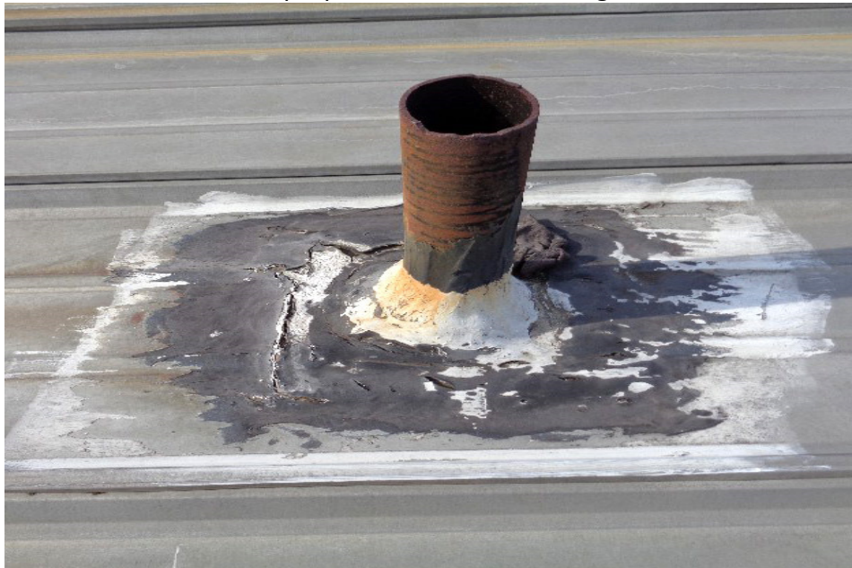
Improper Penetration Flashing
