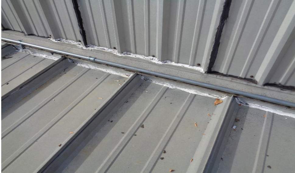
Failed Headwall Flashing
